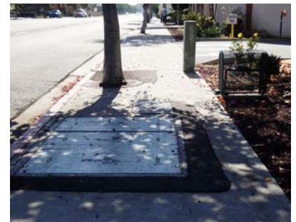
Utility lids and boxes create uneven surfaces, making it difficult to walk and roll
